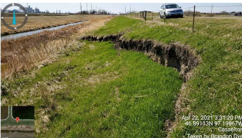
Figure 1. Existing slope sloughing (looking west)
