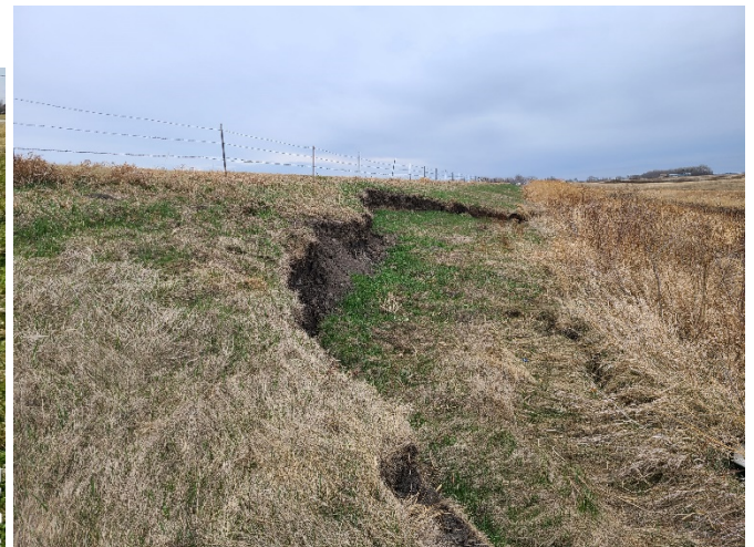
Figure 2. Existing slope sloughing (looking east)
